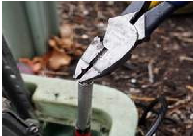
Installation of fiber optics will allow Buckeye CableSystem to deliver more bandwidth for future services such as better high-definition or even 3-D television. Officials of Kabel-X USA said the Perrysburg Township project is the nation's first large-scale test of the technology. ( THE BLADE/AMY E. VOIGT )
