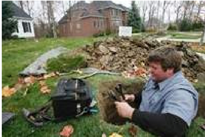
Kenny Mohr, a technician with Kabel-X USA, prepares cable lines in the Carrington Woods subdivision off West River Road for fiber-optic lines to be installed. The process prevents trenching. ( THE BLADE/AMY E. VOIGT )
